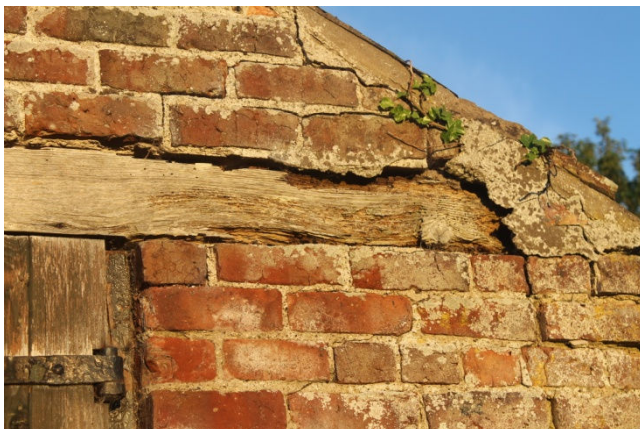
Figure 14: Showing example of gaps associated with the rotten wooden lintel.
