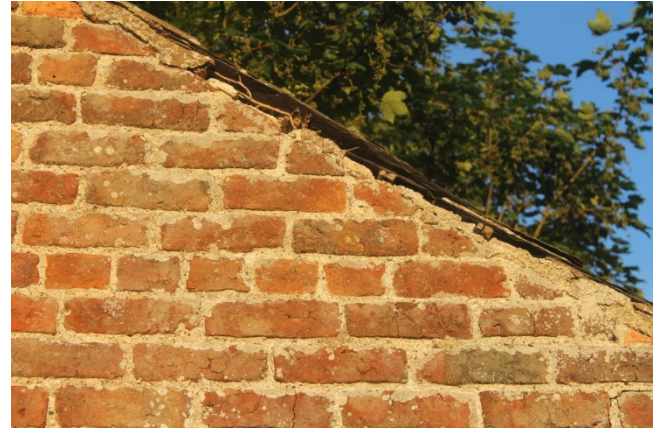
Figure 11: Showing example of gaps at the wall top where cement packing has fallen away at the verges.
