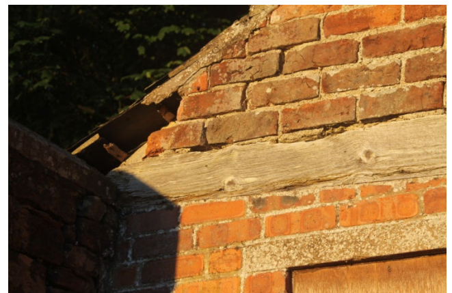
Figure 13: Showing example of wall top gaps.
